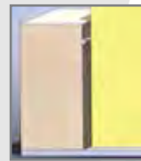
Cable running along the side of ceiling joist with the top of joist not covered in insulation
