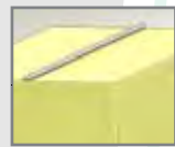
Cable running across the top of a plasterboard ceiling which is covered with thermal insulation
