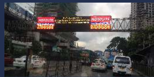
▲ LED traffic signboard
