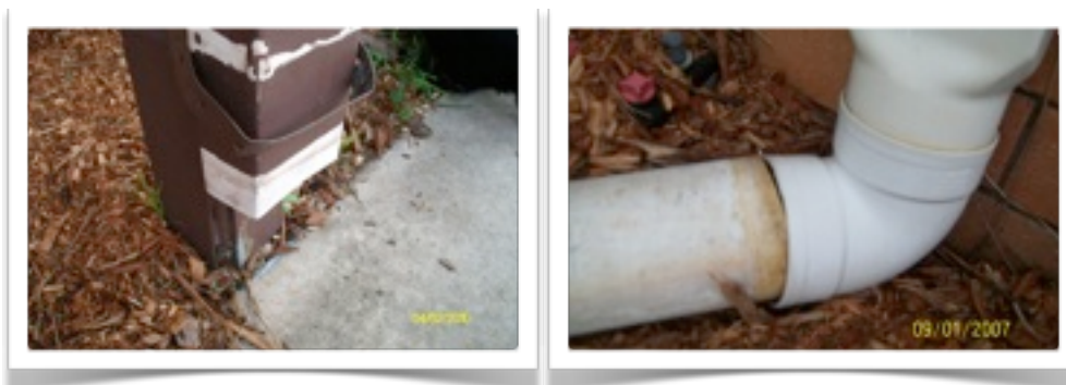
Downpipes discharge direct to ground and should connect to stormwater system
