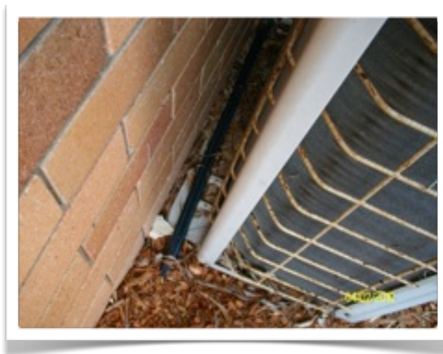
Condensation line discharges direct to ground
