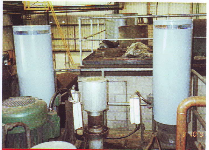
ELECTRIC MOTOR MUFFS INSTALLED ON HYDRAULIC PUMPS
