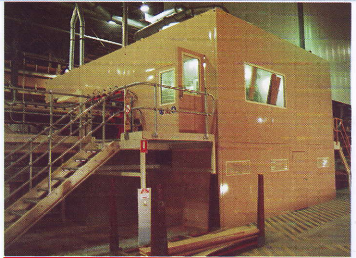
ACOUSTIC ENCLOSURE FOR TRIM SAW AT CSR OBERON
