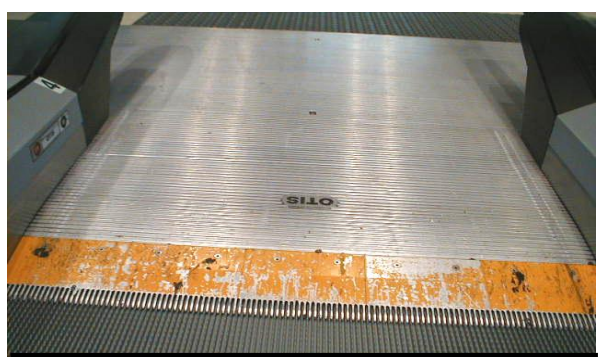
Comb Plate > Due to Impact
