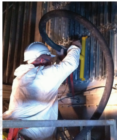
Dust Collector Servicing
