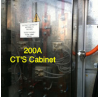
200A CT'S Cabinet
