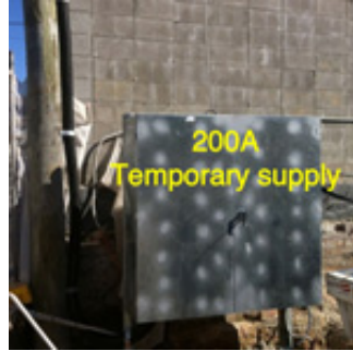
200A Temporary supply
