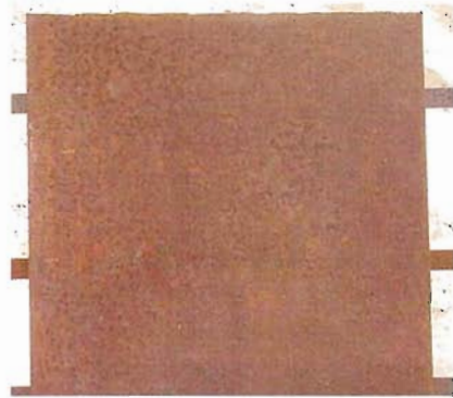
ABOVE ▲ Figure A. The base plate with moderate to heavy rusting.
