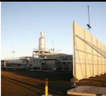
Dalby compressor station upgrade
