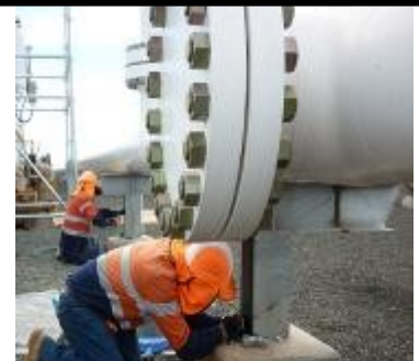
Experienced team of electricians
