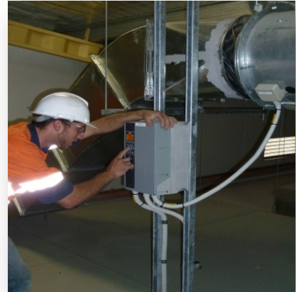
Raphael Muller tests one of three new new variable speed drives that were installed at Cadia East to ensure the project complied with section J BCA criteria
