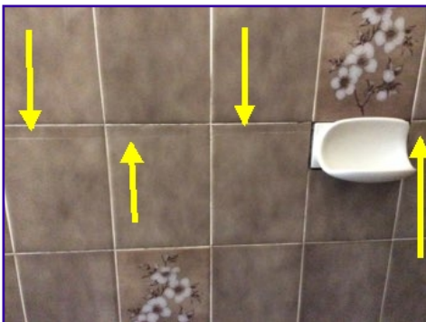
this is the same crack continuing around the shower wall
