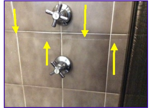
this crack continues around most of the shower, this must be repaired to prevent moisture penetrating behind the tiles and damaging the wall, houses of this age have no waterproofing in wet areas, keeping the tiles and silicone in good order is a must to stop water damage to walls.
