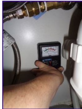
low moisture reading on wall below sink
