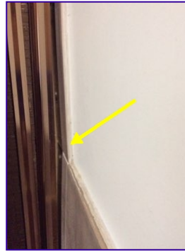
wall is deformed, looks as though it has been pushed and broken, someone has possibly fallen and knocked the wall, therefore damaging it.
