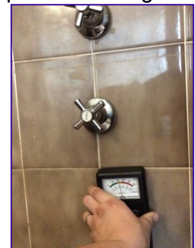
slightly elevated moisture reading
