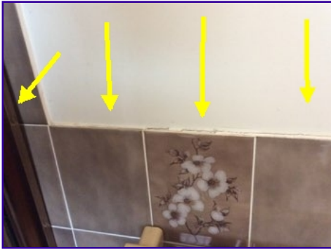
tiles are coming away from wall, this will allow moisture behind tiles, this has already occurred as tiles are drummy and peeling away from walls
