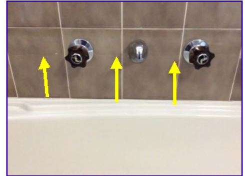
crack which passes through several tiles, this must be repaired to assure no moisture gets behind tiles
