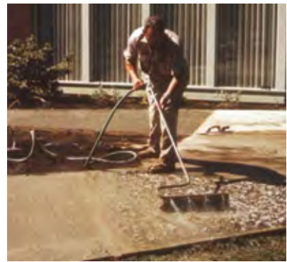
Figure 27 Surface mortar is removed with a stiff-bristled broom, followed by brushing and flushing with a water spray. Shown here is a purpose-made broom with built-in water jets. Brushing and washing continues until the water runs clear and there is no noticeable cement film on the aggregate
