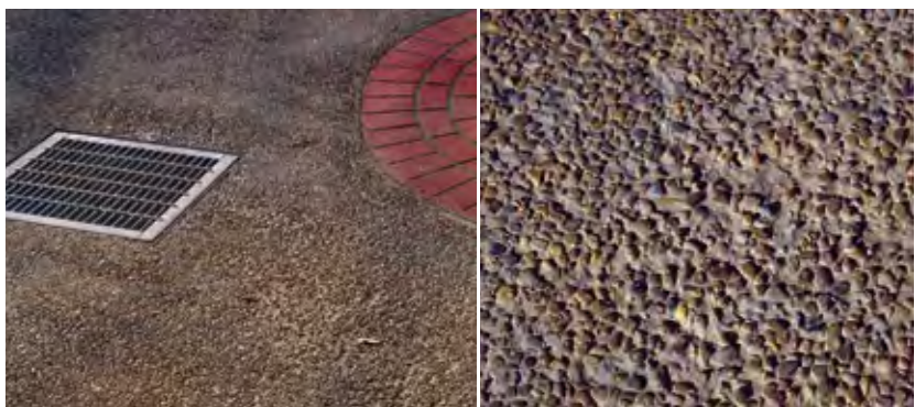
Figure 29 Stones near drain exposed to greater depth by water runoff and subsequently easily dislodged by traffic
