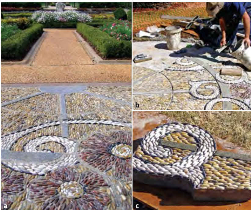
Figure 20 Pebble mosaic formed from smaller precast elements in Parterre Garden, Queens Park, Toowoomba (Artist: Naomi Hatt) [a] Completed work [b] Installing precast sections [c] Individual precast section
