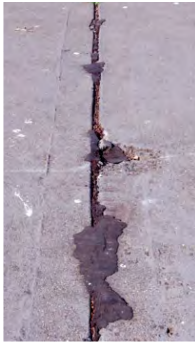
Figure 48 Bitumen squeezed out of joint and spalling along joint from ingress of debris
