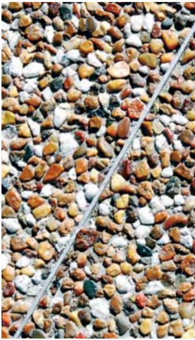
Figure 44 Crack inducer (zinc strip) used to avoid sawcutting at an early age
