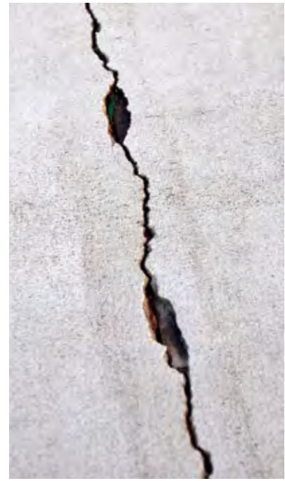
Figure 49 Crack inducer not flush with surface of slab
