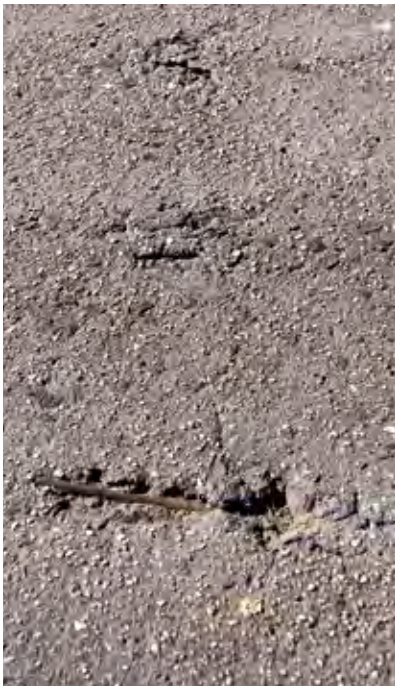
Figure 41 Exposed reinforcement due to inadequate cover
