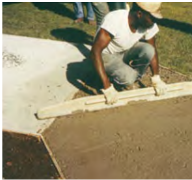
Figure 23 The surface is screeded and bullfloated, generally to the finishes level, although it may be necessary to screed the surface 3–10 mm below the final level to allow for the addition of the aggregate, depending on the size and quantity of stone
