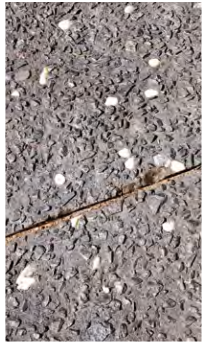
Figure 43 Aggregate particles dislodged during sawcutting
