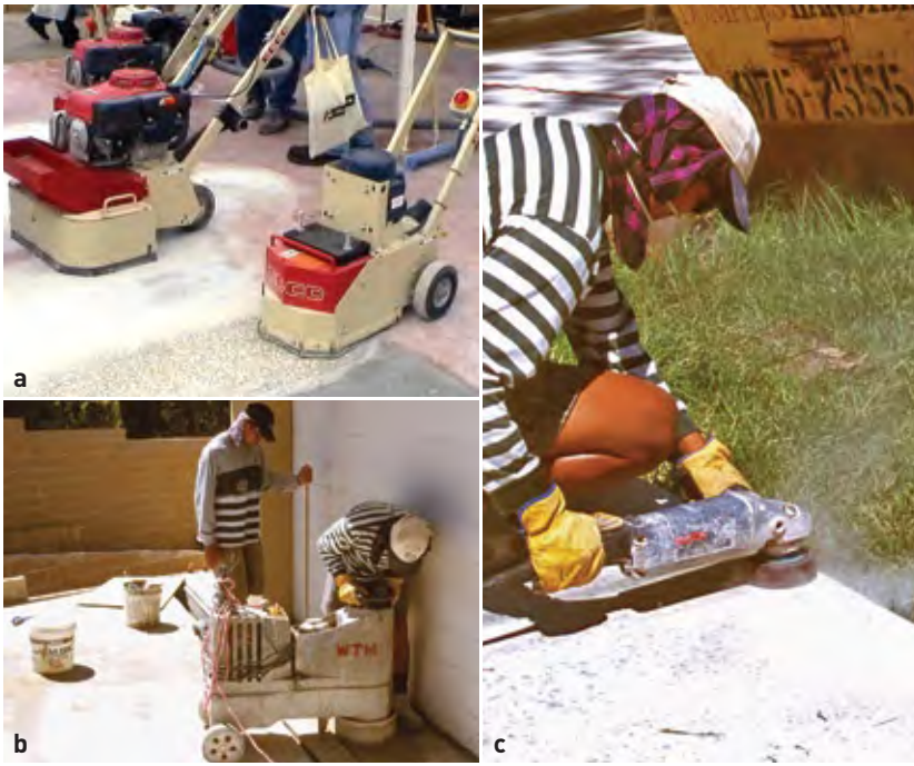
Figure 38 Methods of honing concrete surfaces [a] Dry process [b] Wet process [c] Hand tools for edges
