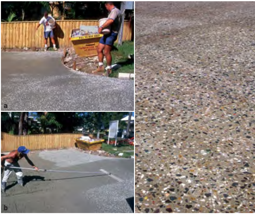
Figure 15 Seeding of selected aggregates [a] Selected aggregates being seeded onto the surface of the concrete after screeding [b] Aggregates being bullfloated into the concrete surface [c] Finished appearance after honing of the surface
