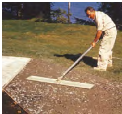
Figure 26 Further embedment is done with bullfloats, as shown here, and hand floats to fully cover the aggregate with the cement matrix (mortar)
