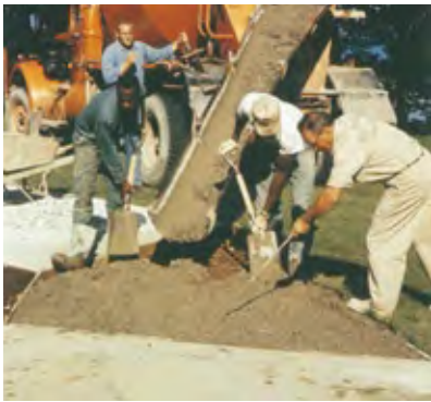
Figure 22 Concrete to be 'seeded' with selected coarse aggregate should have an optimum slump of 100 mm. It is placed and compacted in the usual way
