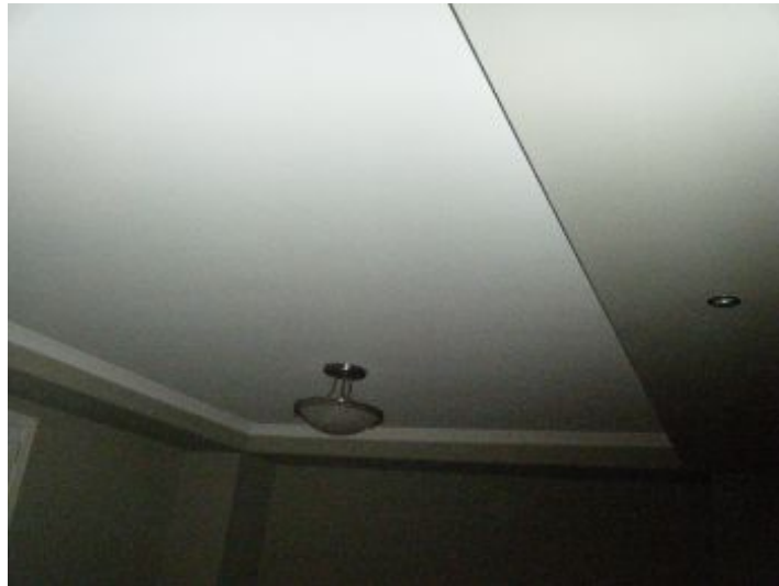
Light not working
