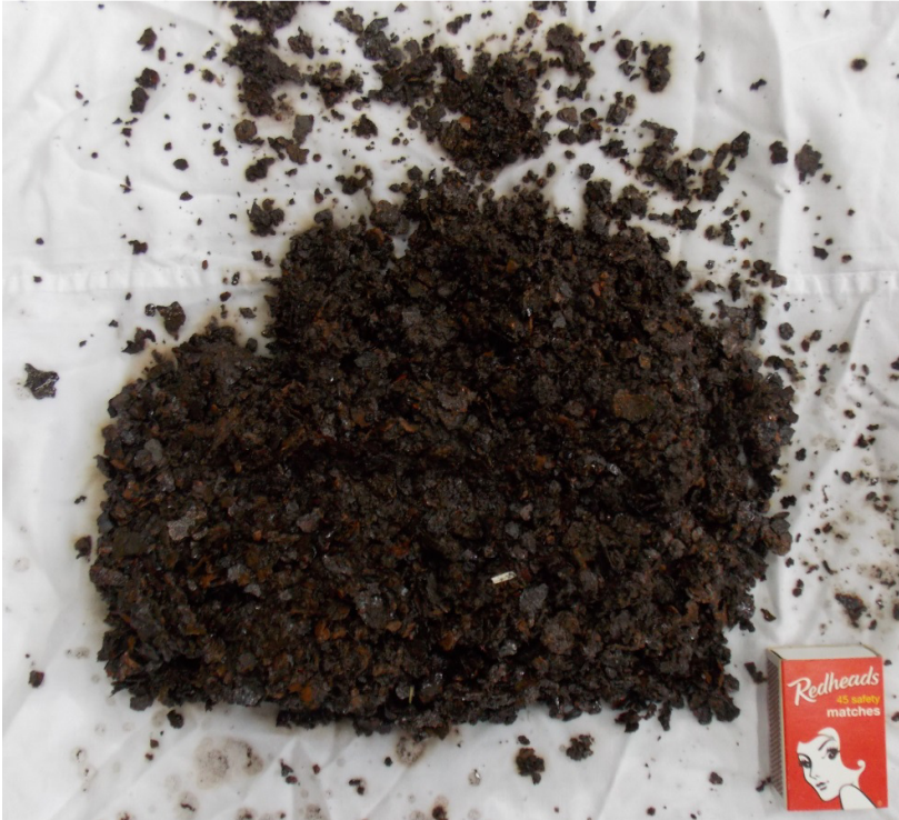
A small amount of the rust removed from the pre-filter.
